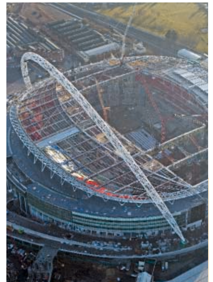
Schindler is supplying escalators for the new Wembley stadium in North London
